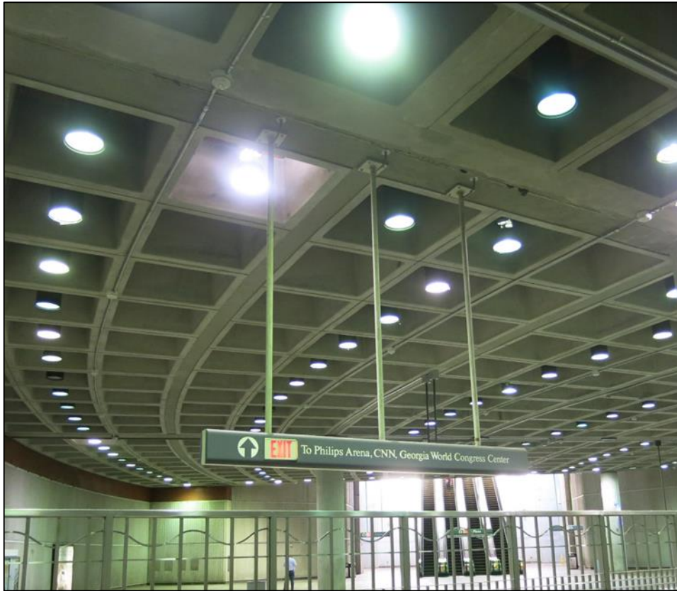
Metal halide lights
